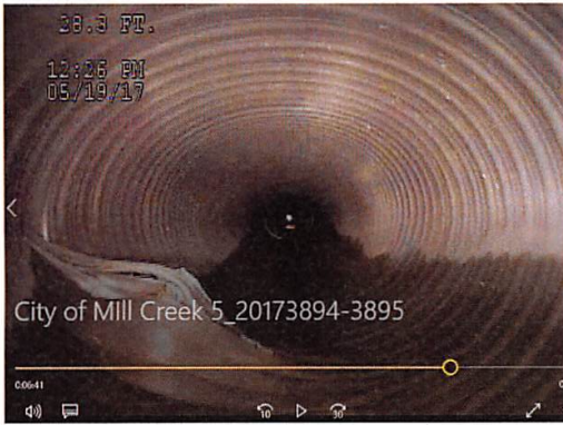
1. Pipe deformation at invert
